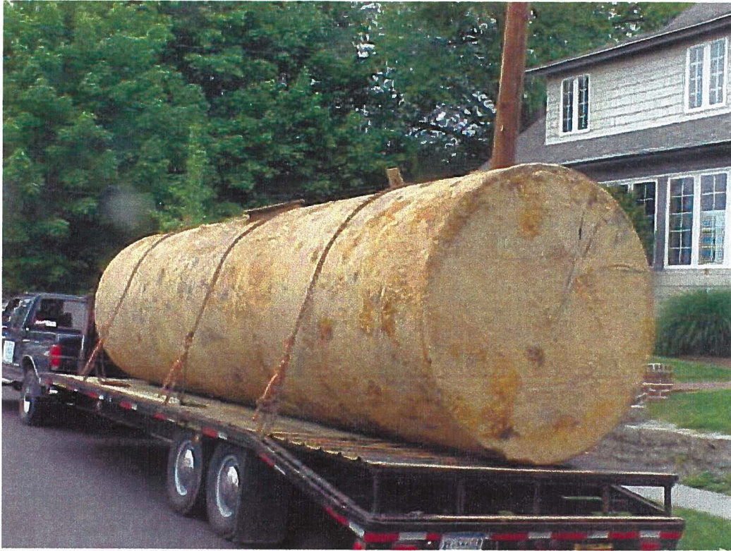
Chevy Chase Branch, DC Public Library – 5,000 gal. UST loaded on trailer for removal
