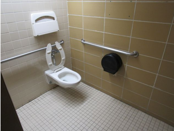
Restroom Fixtures - Single Restrooms Restroom Fixtures - Single Restrooms March 27, 2021
