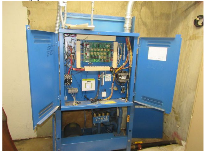
Hydraulic Elevator Hydraulic Elevator March 27, 2021
