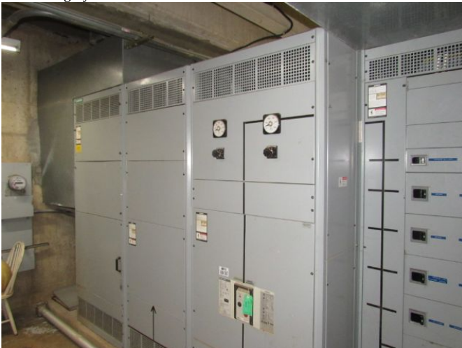
Main Distribution Switchboard - 2500A 480/277V 3 phase Main Distribution Switchboard - 2500A 480/277V 3 phase March 27, 2021
