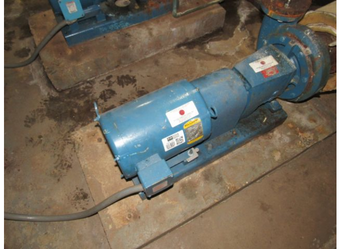
HVAC Pump - Chilled / Hot Water - Base-Mounted (P2) - 10 HP HVAC Pump - Chilled / Hot Water - Base-Mounted (P2) - 10 HP March 27, 2021
