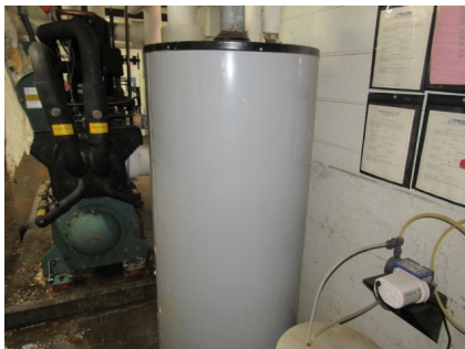
Water Heater - Gas - Comm - 100 Gallons
