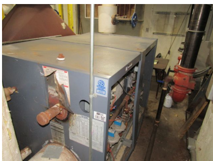
Boiler - Cast Iron Sectional - 1690 MBH (# 1)
