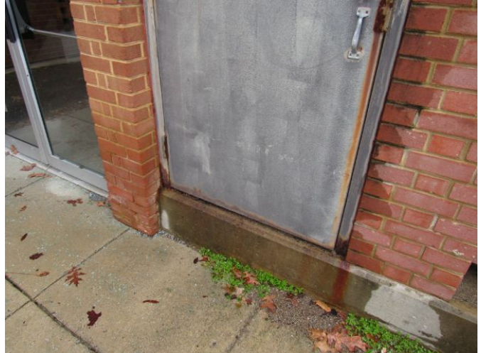
Door Assembly - Single - Hollow Metal (Roof + Generator Enclosure) Door Assembly - Single - Hollow Metal (Roof + Generator Enclosure) March 27, 2021
