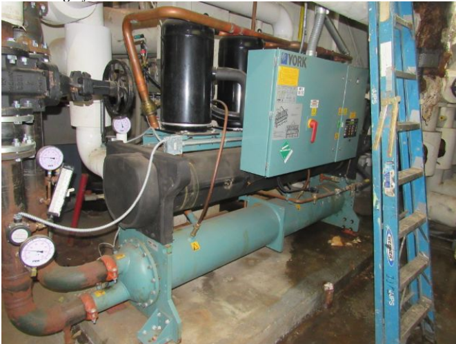
Chiller - Scroll - 94 Ton Chiller - Scroll - 94 Ton March 27, 2021
