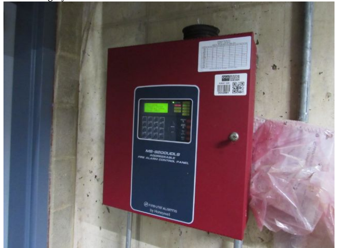
Fire Alarm System - FACP Fire Alarm System - FACP March 27, 2021
