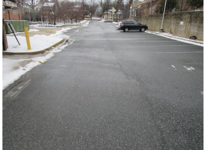
Asphalt Parking Lot - Life Cycle Maintenance - East Elevation Asphalt Parking Lot - Life Cycle Maintenance - East Elevation March 27, 2021
