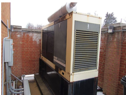
Emergency Generator - 80kW - Diesel
