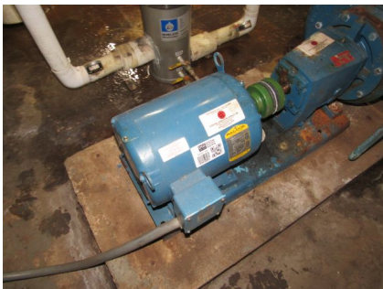
HVAC Pump - Chilled / Hot Water - Base-Mounted (P1) - 7.5 HP
