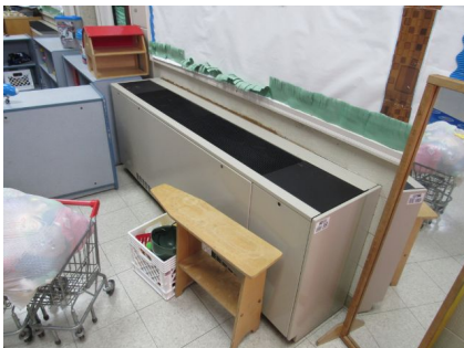
Vertical Fan Coil Floor Mounted (100") - (Original Installation)
