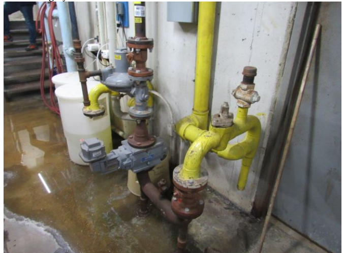
Natural Gas Supply for Bldg - 3" Feed Natural Gas Supply for Bldg - 3" Feed March 27, 2021
