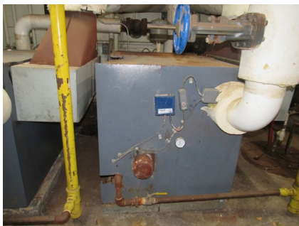
Boiler - Cast Iron Sectional - 1690 MBH (# 2)
