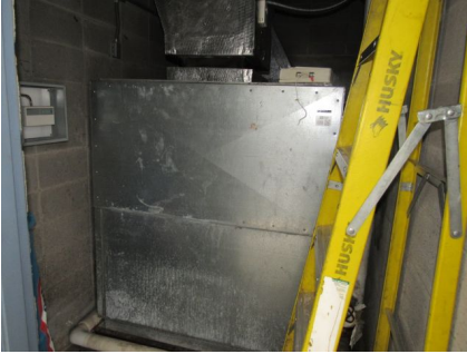
Air Handling Unit - Single Zone, Low Pressure Central Station (AHU 5) - 2,000 CFM
