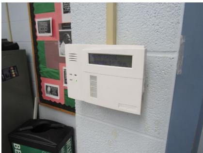
Security System - Intrusion Alarm
