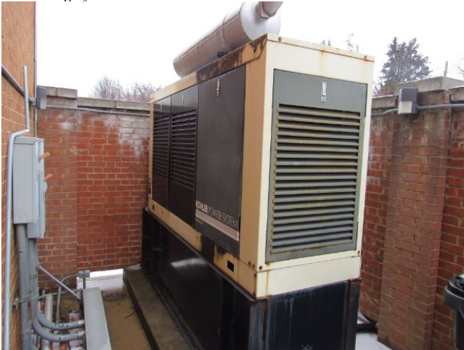
Emergency Generator - General Wear - At-Grade Emergency Generator - General Wear - At-Grade March 27, 2021
