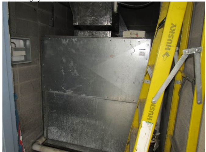
Air Handling Unit - Single Zone, Low Pressure Central Station (AHU 5) - 2,000 CFM Air Handling Unit - Single Zone, Low Pressure Central Station (AHU 5) - 2,000 CFM March 27, 2021
