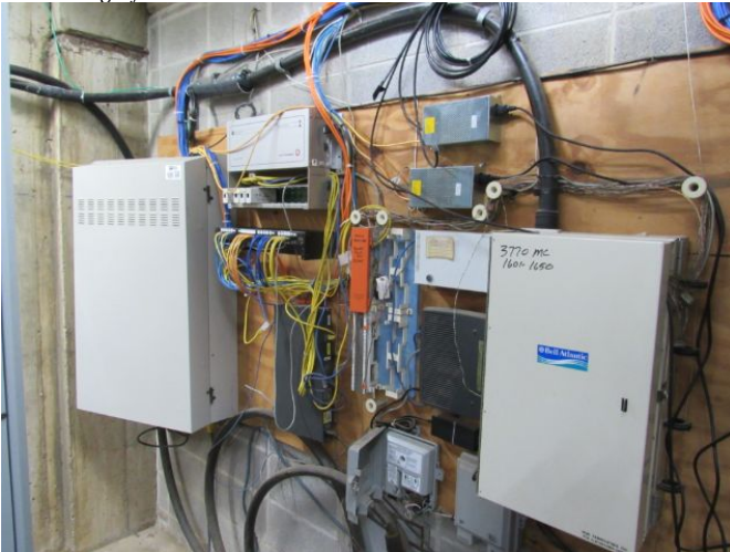
Telephone System Telephone System March 27, 2021
