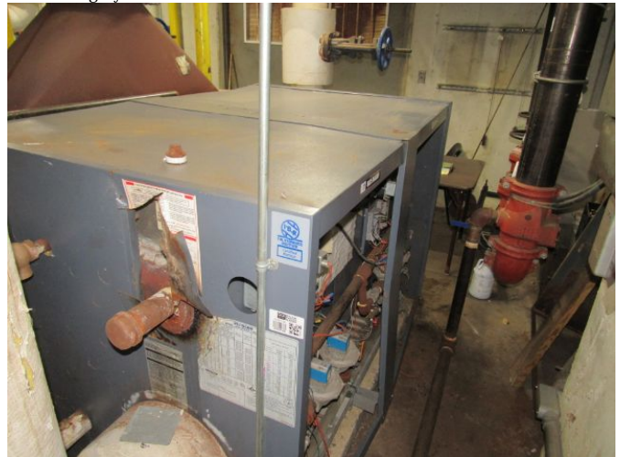
Boiler - Cast Iron Sectional - 1690 MBH (# 1) Boiler - Cast Iron Sectional - 1690 MBH (# 1) March 27, 2021
