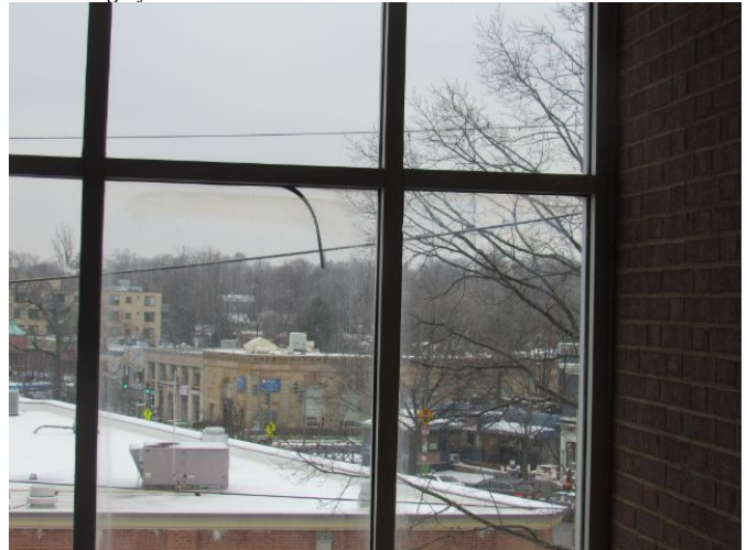
Aluminum Windows Detached Window Gasket March 27, 2021
