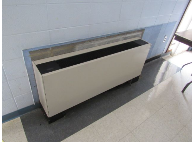
Vertical Fan Coil Floor Mounted (56") - (1999 Installation) Vertical Fan Coil Floor Mounted (56") - (1999 Installation) March 27, 2021
