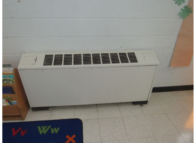
Vertical Fan Coil Floor Mounted (56") - (Original Installation) Vertical Fan Coil Floor Mounted (56") - (Original Installation) March 27, 2021
