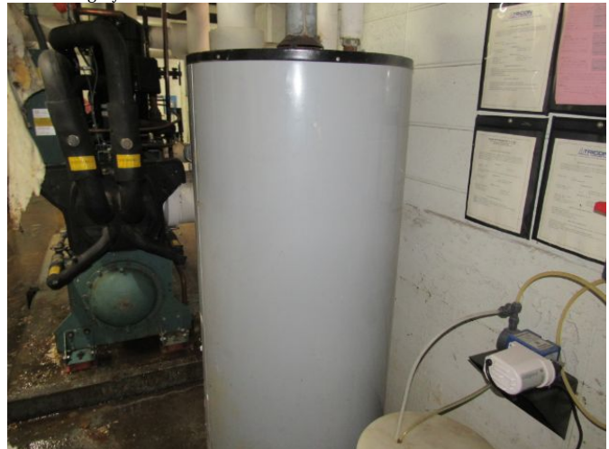
Water Heater - Gas - Comm - 100 Gallons Water Heater - Gas - Comm - 100 Gallons March 27, 2021
