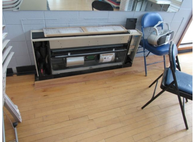
Vertical Fan Coil Floor Mounted (56") - (1999 Installation) Vertical Fan Coil Floor Mounted (56") - (1999 Installation) March 27, 2021
