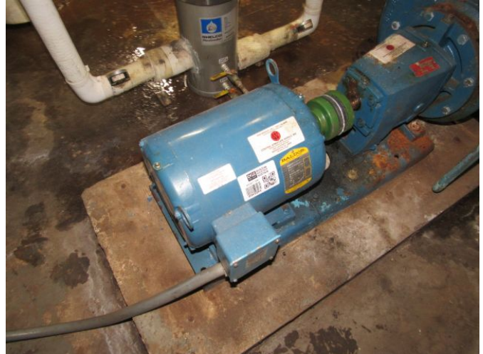
HVAC Pump - Chilled / Hot Water - Base-Mounted (P1) - 7.5 HP HVAC Pump - Chilled / Hot Water - Base-Mounted (P1) - 7.5 HP March 27, 2021
