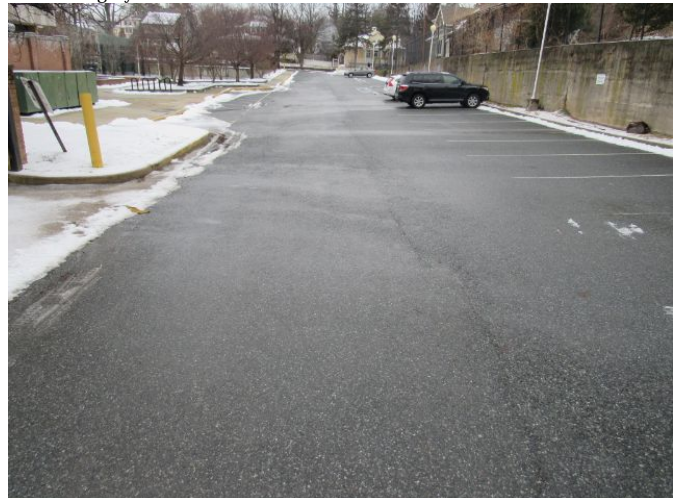
Asphalt Parking Lot & Roadway - Wearing Surface Will Exceed Life - East Elevation Asphalt Parking Lot & Roadway - Wearing Surface Will Exceed Life - East Elevation March 27, 2021
