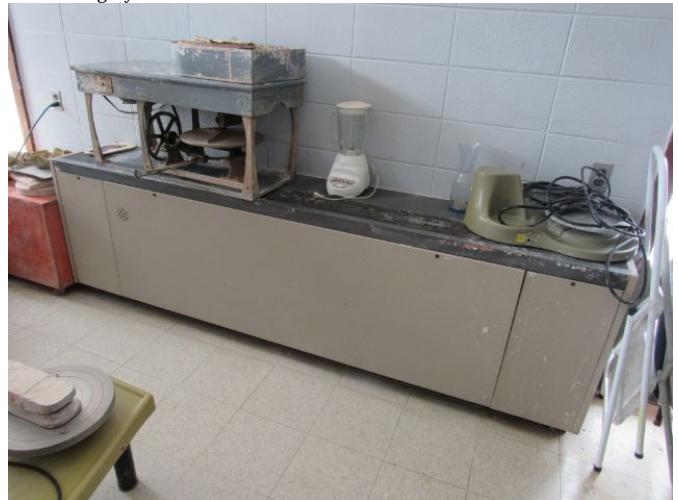
Vertical Fan Coil Floor Mounted (100") - (1999 Installation) Vertical Fan Coil Floor Mounted (100") - (1999 Installation) March 27, 2021
