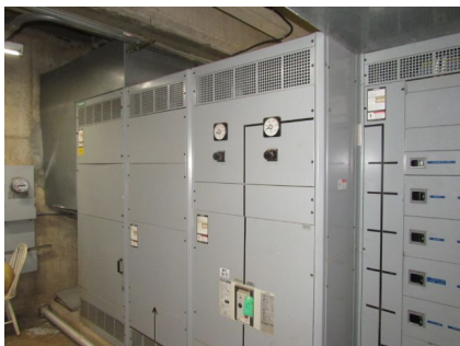
Main Distribution Switchboard - 2500A 480/277V 3 phase
