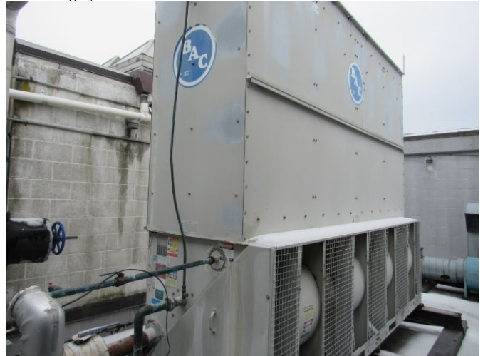
Cooling Tower - Galvanized Steel - 107 Ton Cooling Tower - Galvanized Steel - 107 Ton March 27, 2021
