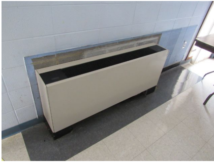
Vertical Fan Coil Floor Mounted (56") - (1999 Installation)
