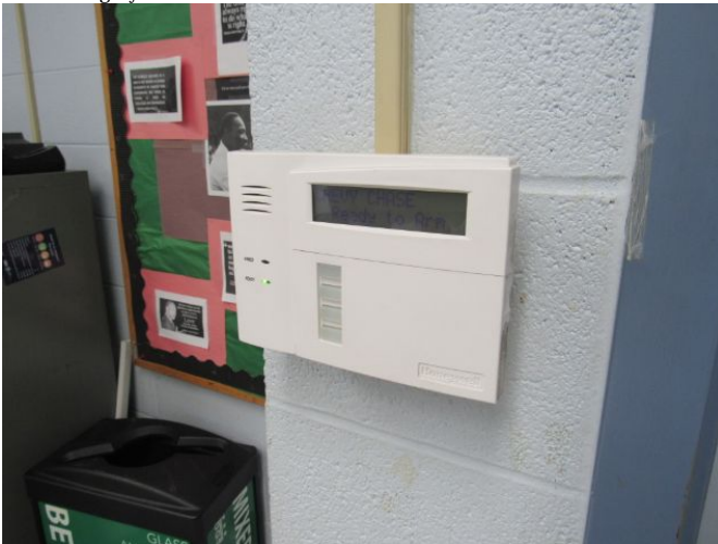
Security System - Intrusion Alarm Security System - Intrusion Alarm March 27, 2021
