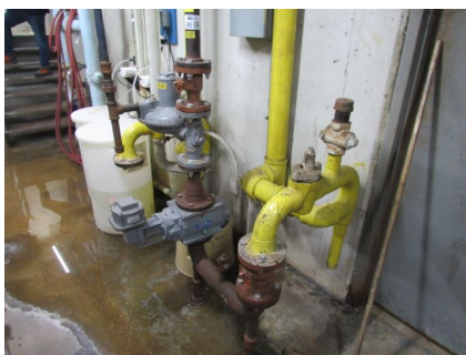
Natural Gas Supply for Bldg - 3" Feed
