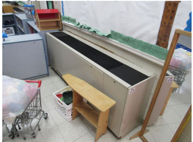
Vertical Fan Coil Floor Mounted (100") - (Original Installation) Vertical Fan Coil Floor Mounted (100") - (Original Installation) March 27, 2021
