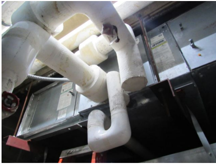
Air Handling Unit - Single Zone, Low Pressure Central Station (AHU 1) - 2,000 CFM
