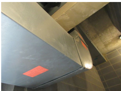
HVAC Ductwork - Supply - Multi-Zone
