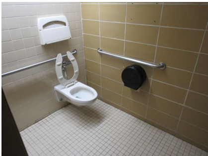
Restroom Fixtures - Single Restrooms
