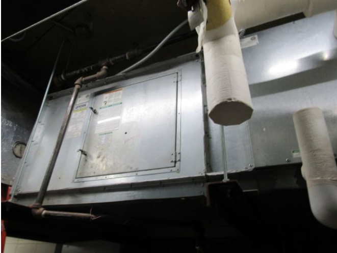
Air Handling Unit - Single Zone, Low Pressure Central Station (AHU 3) - 2,000 CFM Air Handling Unit - Single Zone, Low Pressure Central Station (AHU 3) - 2,000 CFM March 27, 2021
