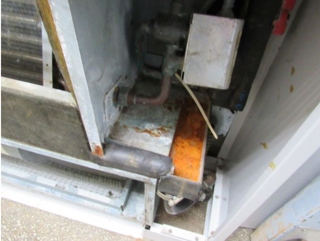
Piping Distribution - 2 Pipe - Hot / Chilled / Condenser Water Piping Distribution - 2 Pipe - Hot / Chilled / Condenser Water March 27, 2021
