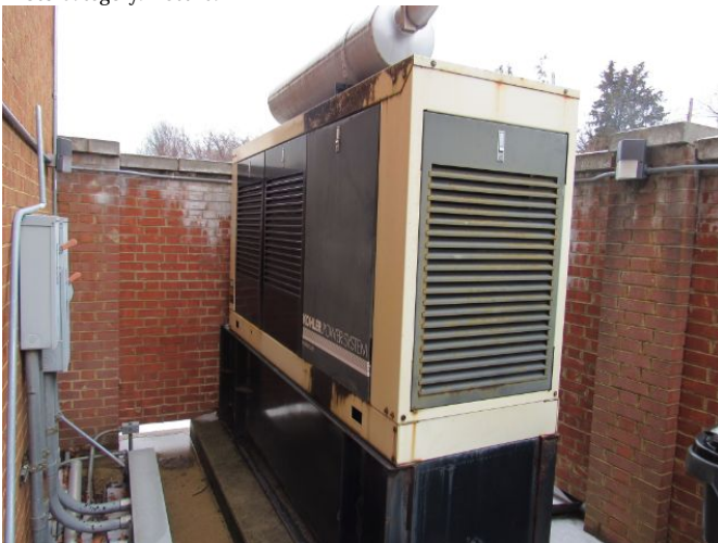
Emergency Generator - 80kW - Diesel Emergency Generator - 80kW - Diesel March 27, 2021
