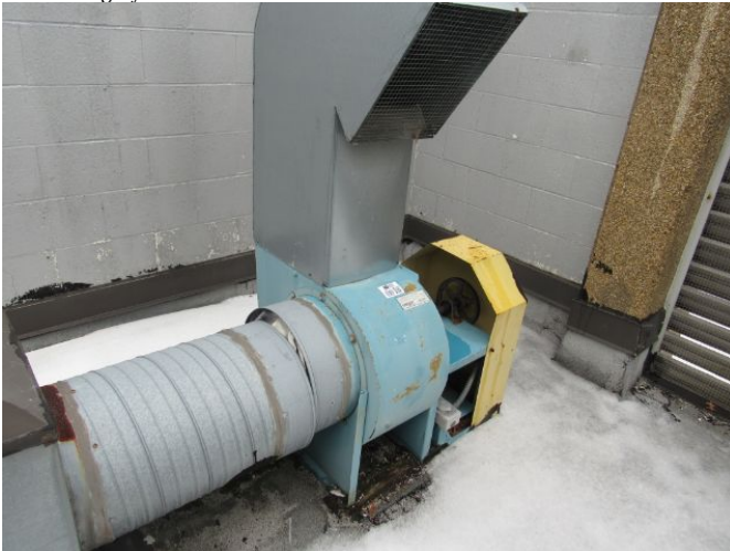
Exhaust Ventilator - Roof - (1,500 CFM) Exhaust Ventilator - Roof - (1,500 CFM) March 27, 2021
