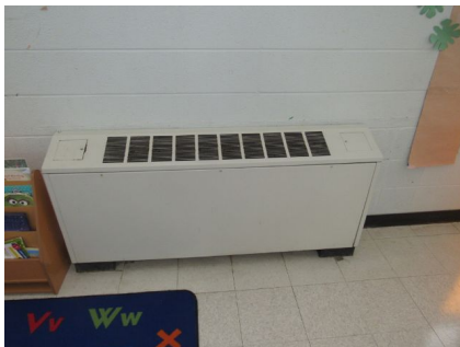
Vertical Fan Coil Floor Mounted (56") - (Original Installation)
