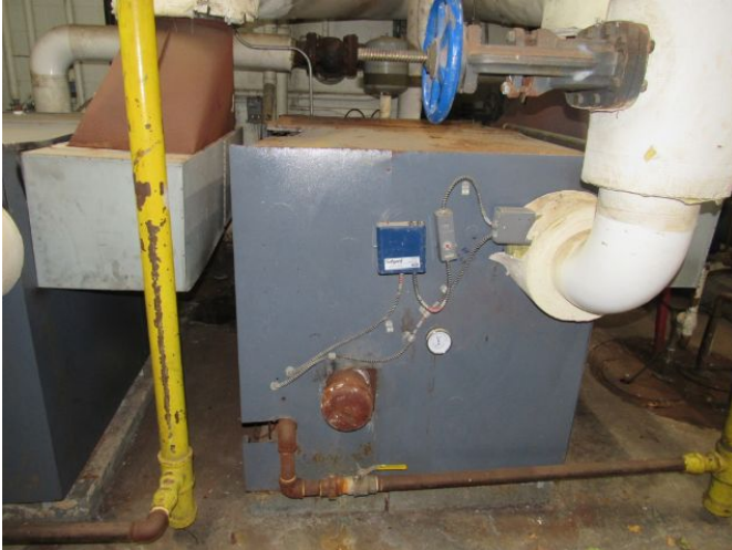
Boiler - Cast Iron Sectional - 1690 MBH (# 2) Boiler - Cast Iron Sectional - 1690 MBH (# 2) March 27, 2021
