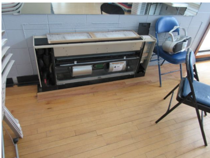
Vertical Fan Coil Floor Mounted (56") - (1999 Installation)
