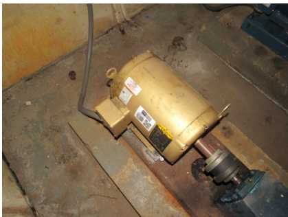
HVAC Pump - Chilled / Hot Water - Base-Mounted (P3) - 10 HP
