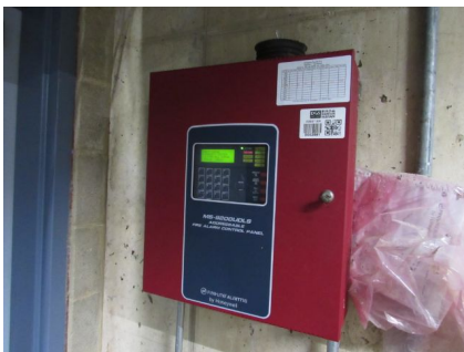
Fire Alarm System - FACP
