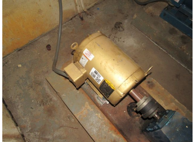
HVAC Pump - Chilled / Hot Water - Base-Mounted (P3) - 10 HP HVAC Pump - Chilled / Hot Water - Base-Mounted (P3) - 10 HP March 27, 2021
