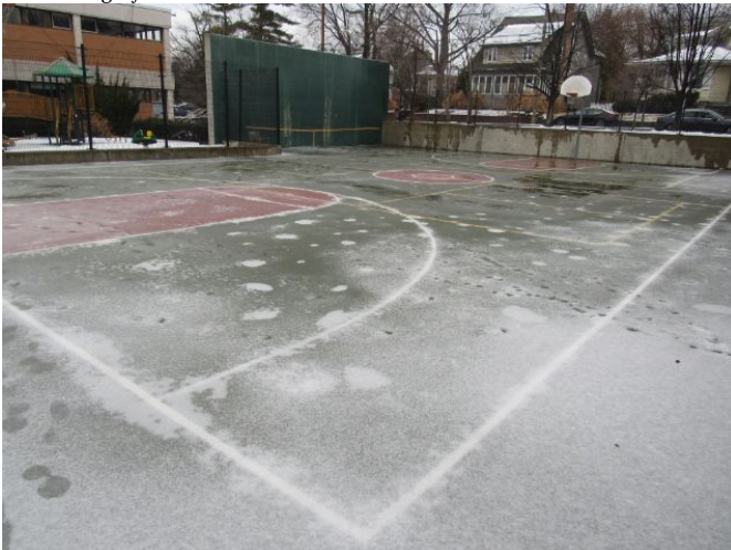
Site Development - Basketball Court - Asphaltic Concrete Site Development - Basketball Court - Asphaltic Concrete March 27, 2021
