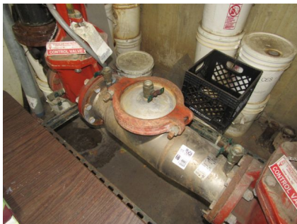
Sprinkler System - Backflow Preventer 6"
