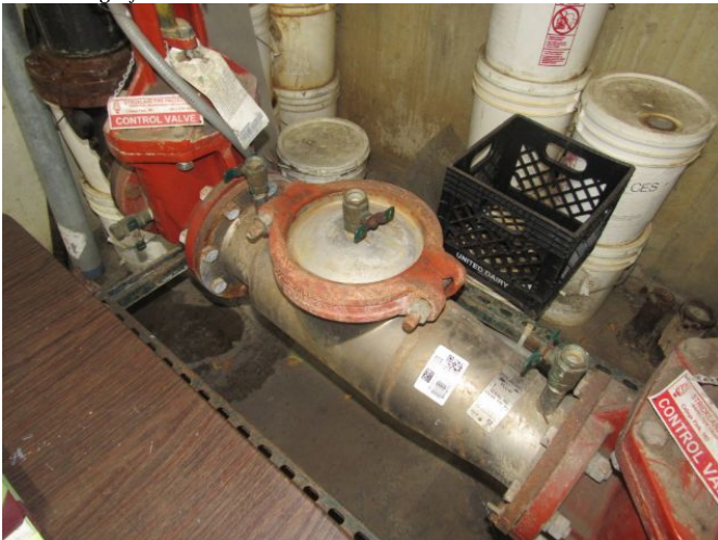
Sprinkler System - Backflow Preventer 6" Sprinkler System - Backflow Preventer 6" March 27, 2021
