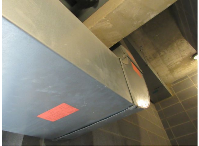
HVAC Ductwork - Supply - Multi-Zone HVAC Ductwork - Supply - Multi-Zone March 27, 2021
