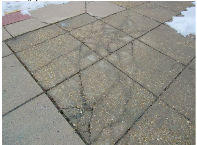
Concrete Sidewalks - Cracked - East Elevation Concrete Sidewalks - Cracked - East Elevation March 27, 2021
