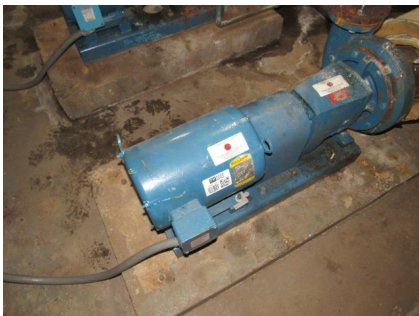
HVAC Pump - Chilled / Hot Water - Base-Mounted (P2) - 10 HP
