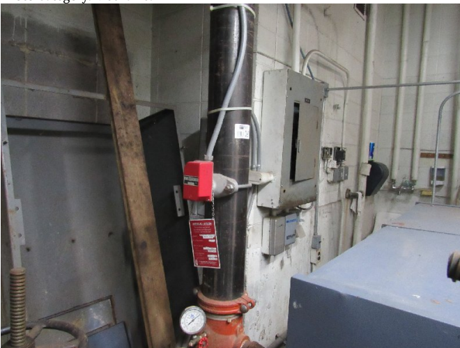
Sprinkler System - Wet - Ordinary Hazard Sprinkler System March 27, 2021
